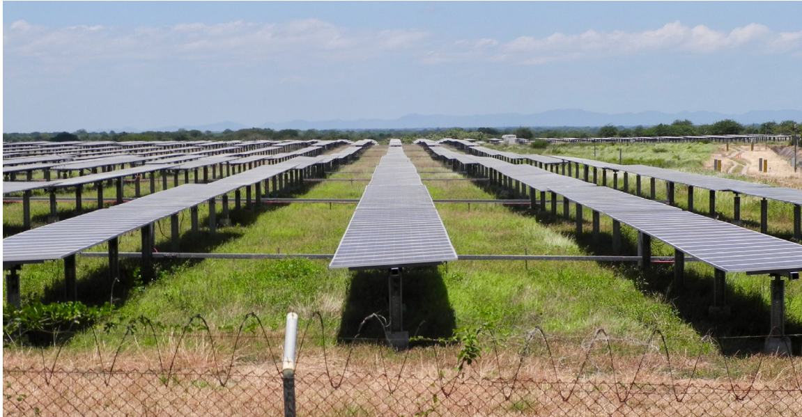
X-Elio's Marcovia Solar Park, southern Honduras; Credit: Jen Moore
